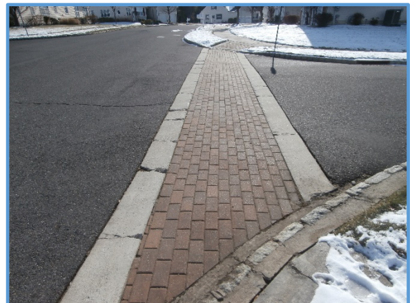
Pre-Cast Concrete Paver Walkway
